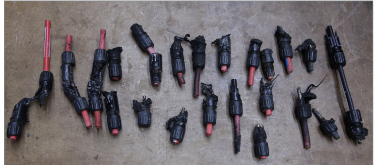
The sample of failed connectors above melted due to high temperature operation in the field. PVEL removed the devices from the field for testing and root cause failure analysis.
