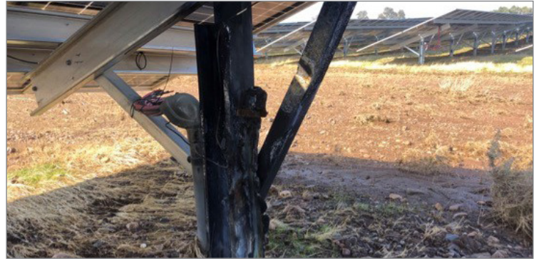
A single overheated connector caused this catastrophic failure. Per PVEL's testing, installation error is likely the root cause.
