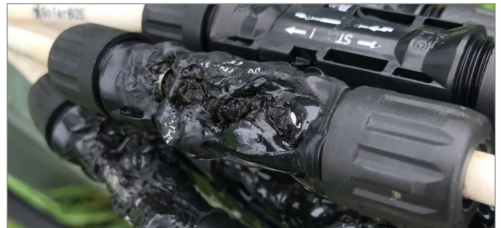
Burnt and melted connectors at an operating project.
