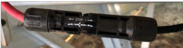
A mismatched MC4 and MC4-compatible connector in the field at a site with extensive connector failures.
