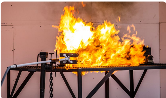
The image above shows a battery energy storage system in thermal runaway during destructive testing.
