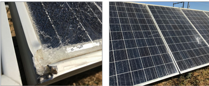
Hail damage at a solar project in California
